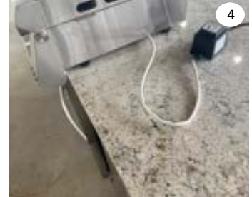
4 Do the same on the other side to ensure the overall flatness and run the power cord to the transformer between the legs.
